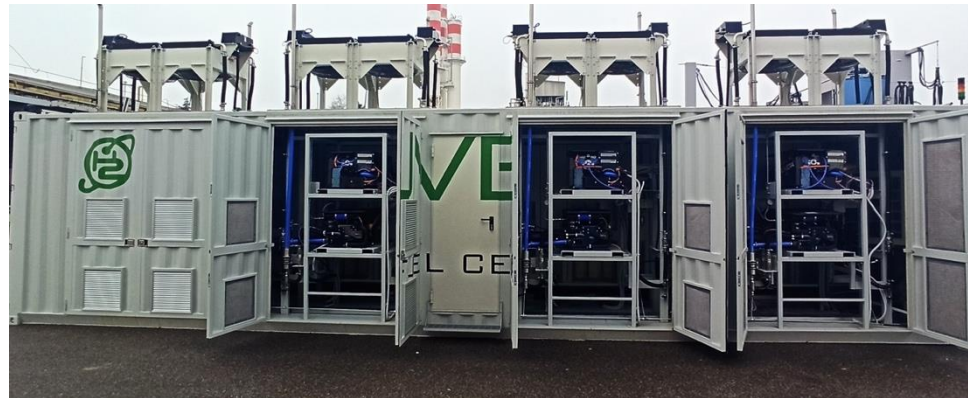
Fuel Cell Durability Test Facility – Osio, Italy
