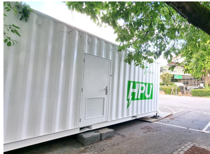
250kW 'HPU Fast' deployed since Jan 2022
