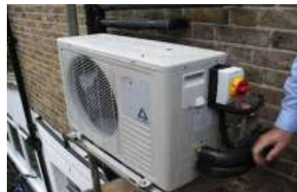
Air source heat pump trial
