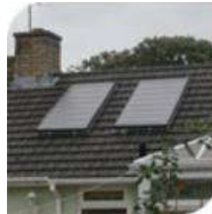
Solar Hot water
